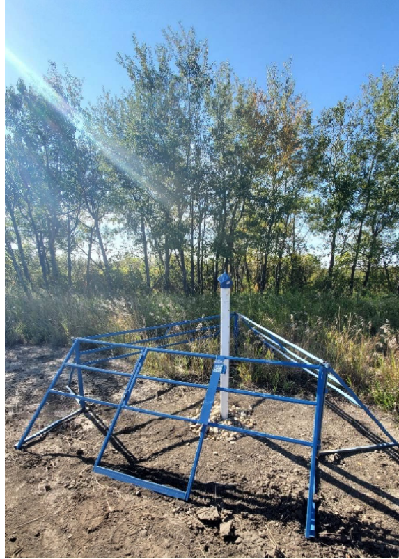
Fig. 9: Produced Water Sensor Installation
